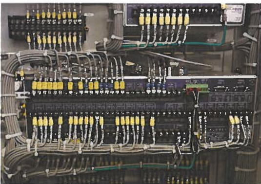
The installation of our customized wiring sets the industry standard for quality and efficiency
