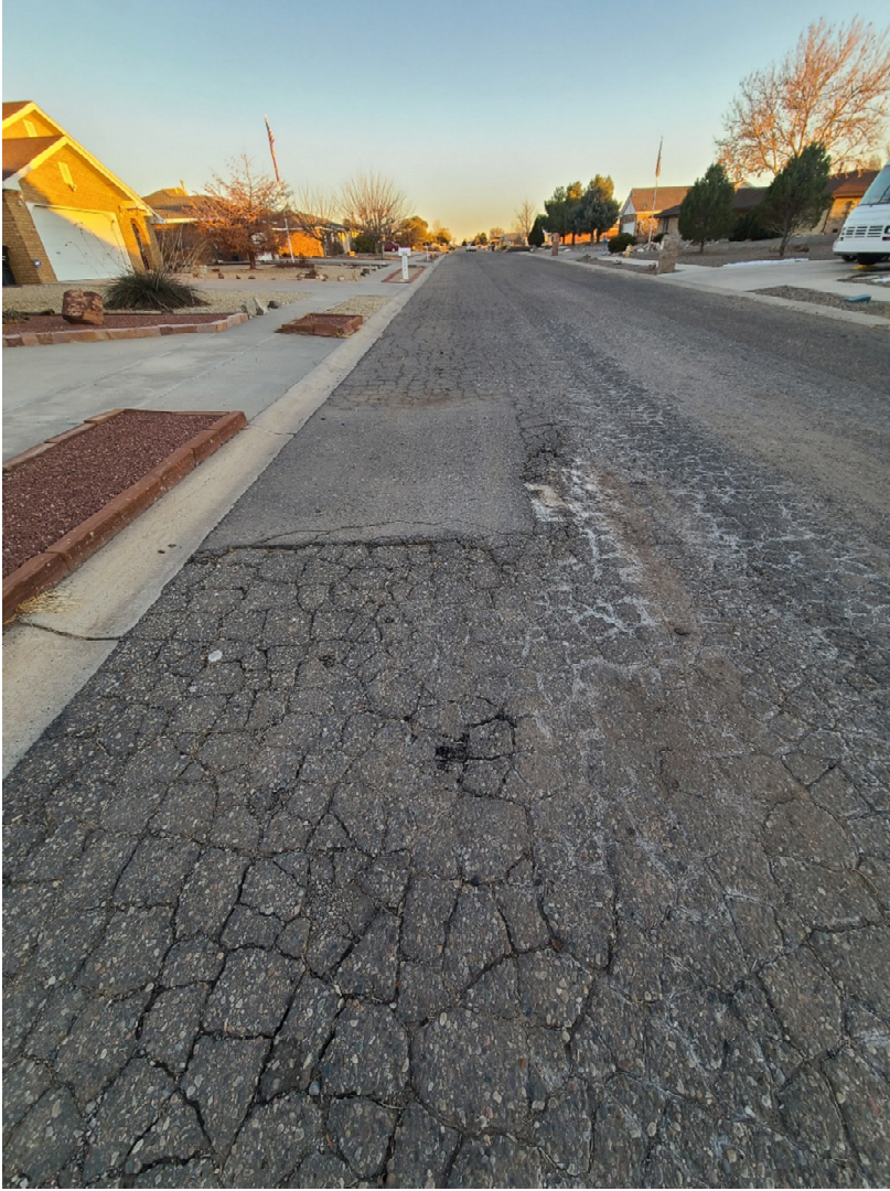
Figure 4: Alligator cracking and subgrade failure
