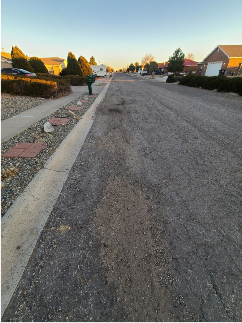
Figure 2: Excessive cracking and subgrade exposure
