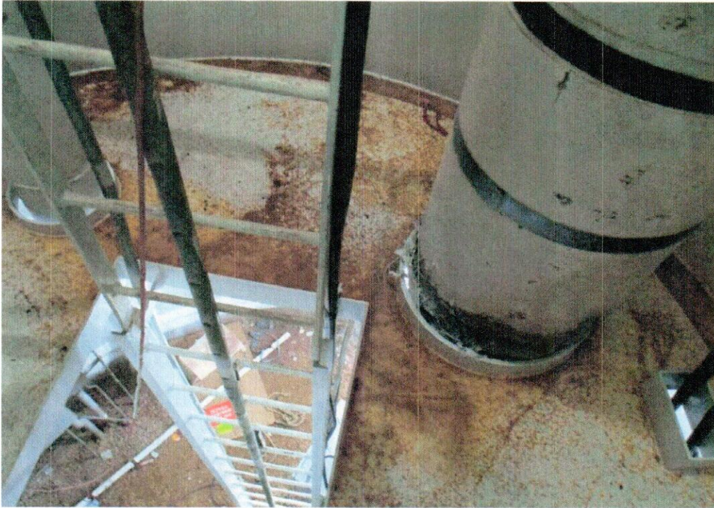
Condensate Platform - Fair Condition - Debris & Staining
