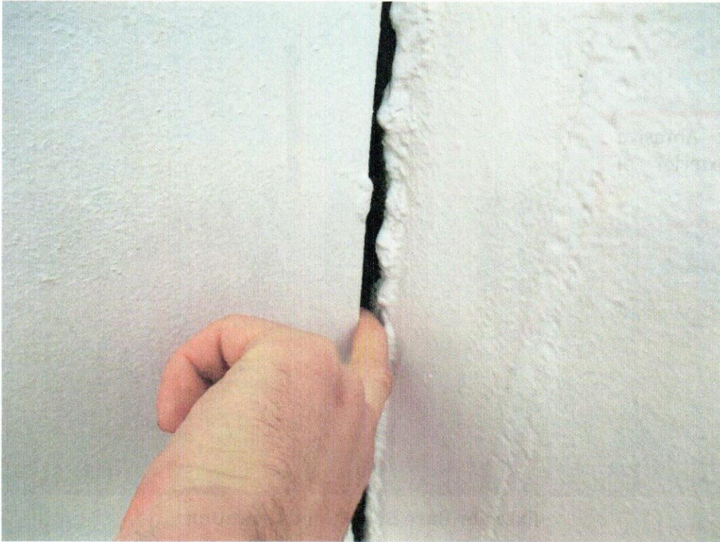
Exterior Base Bell - Gap in Telecom Structure
