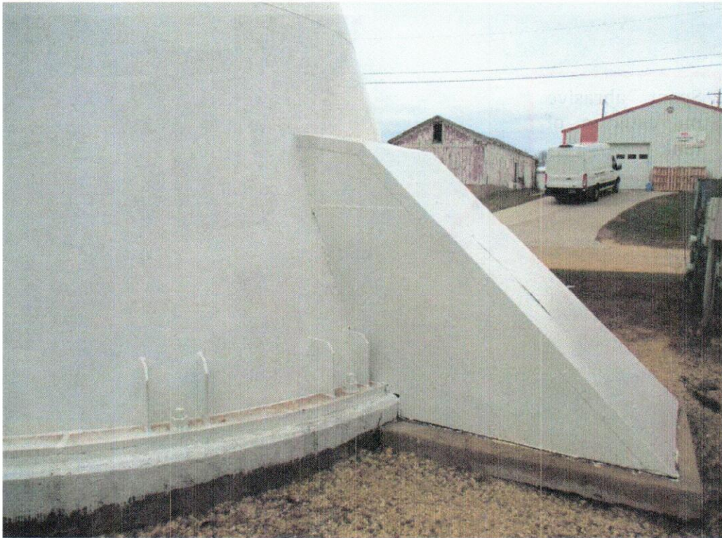
Exterior Base Bell - Gap in Telecom Structure
