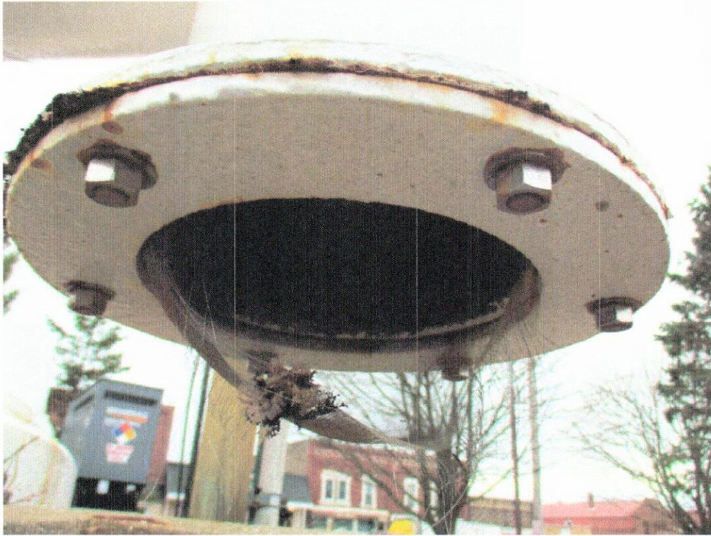
Exterior Overflow – Poor Condition – Broken Mesh
