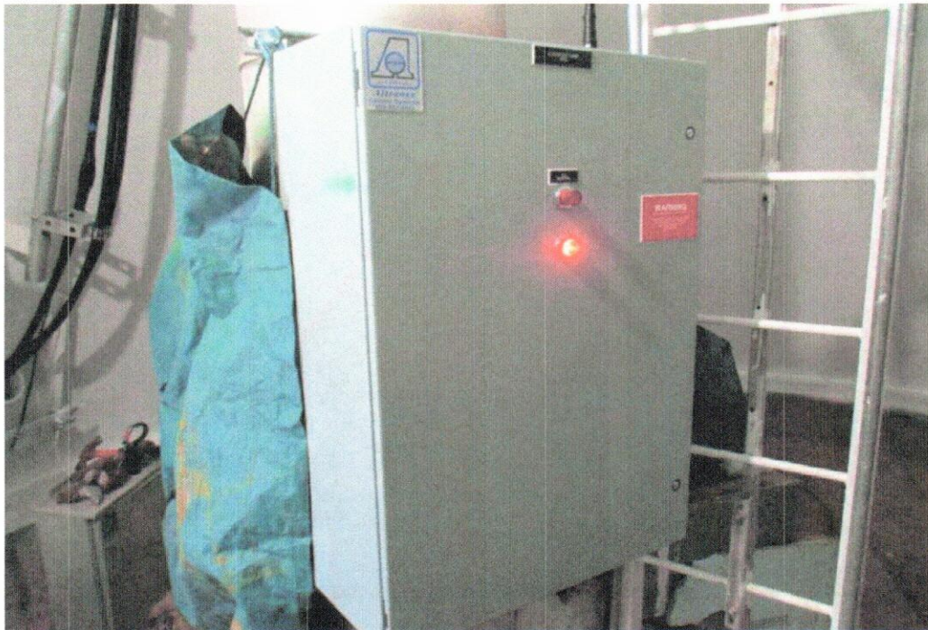
Scada Fill Panel - Good Condition
