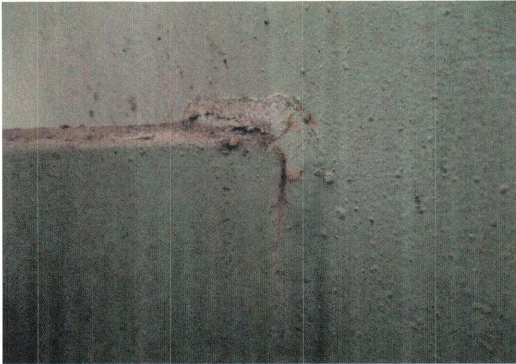
Riser - Coating Crack
