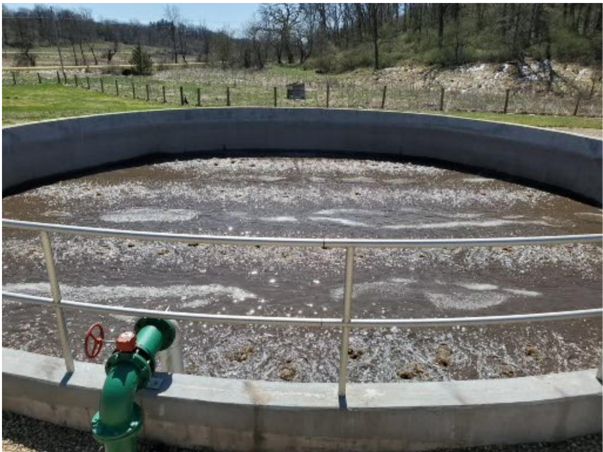
Picture #6 - Aerated Sludge Storage
