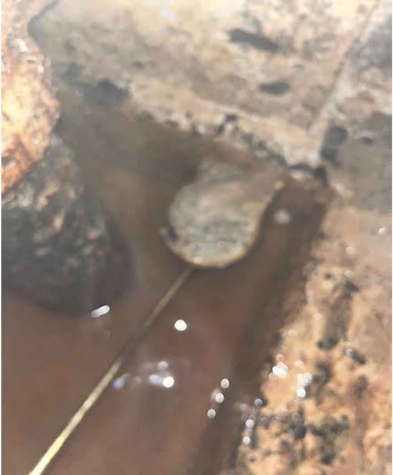
The Sump was Filled with Sediment
