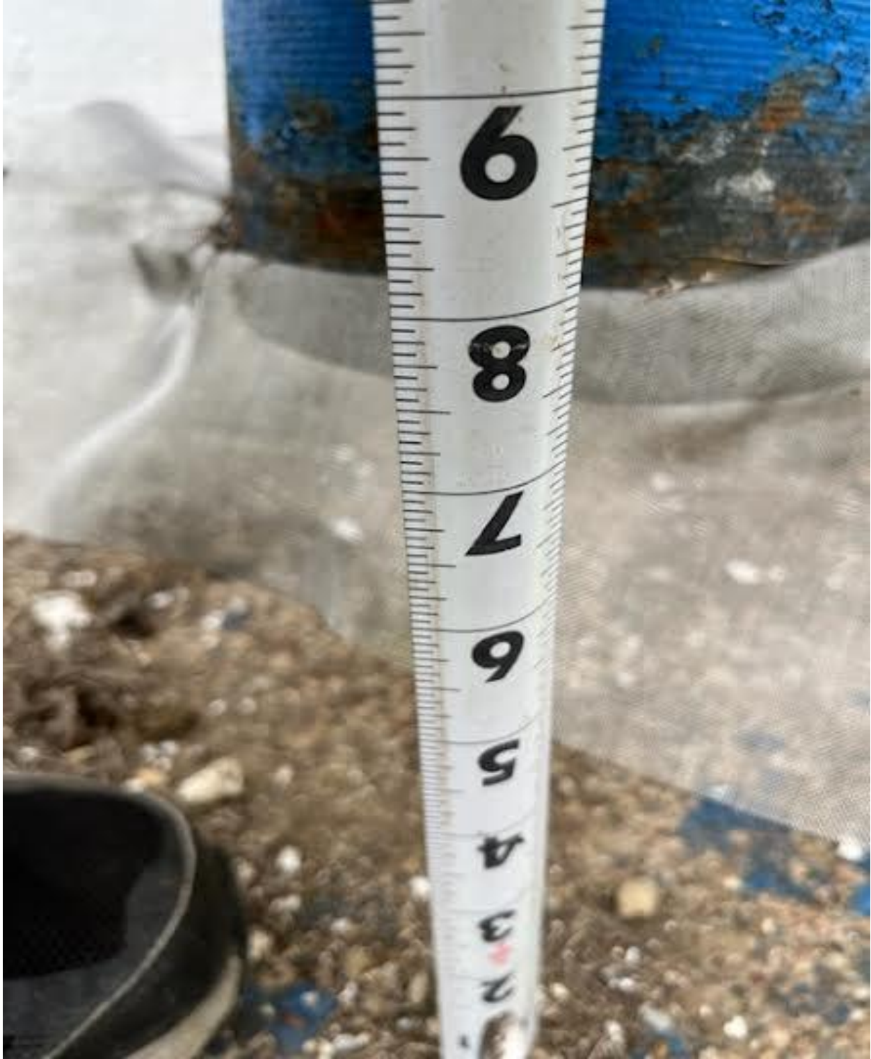
The Overflow Air Gap is at 8"
