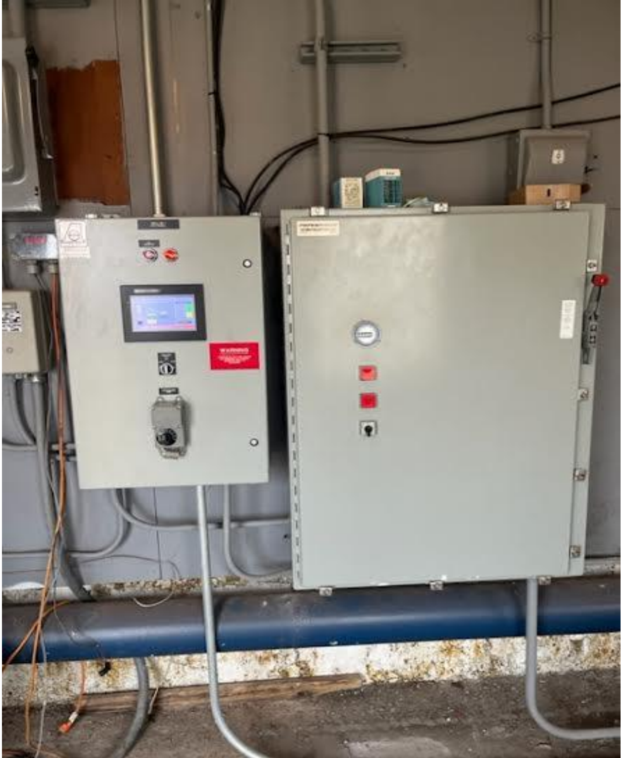
The Electrical and Fill Telemetry
