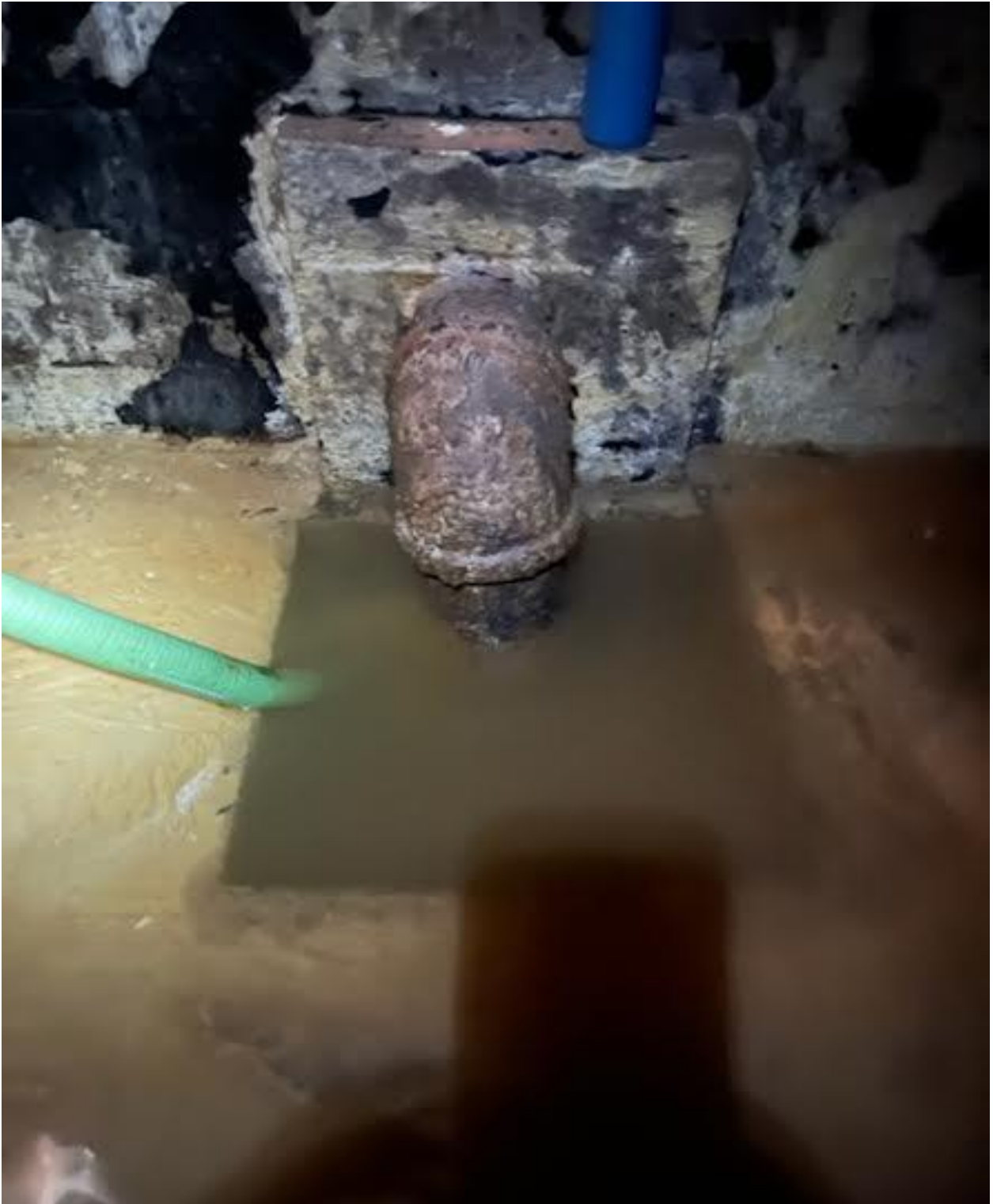
The Outlet Pipe is located in Sump
