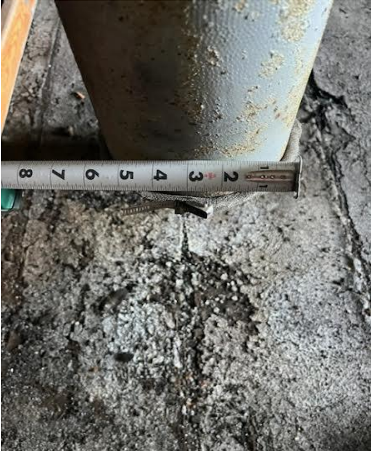
6" Diameter Air Vent
