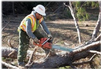
Hazard Tree Removal (Leaner)
