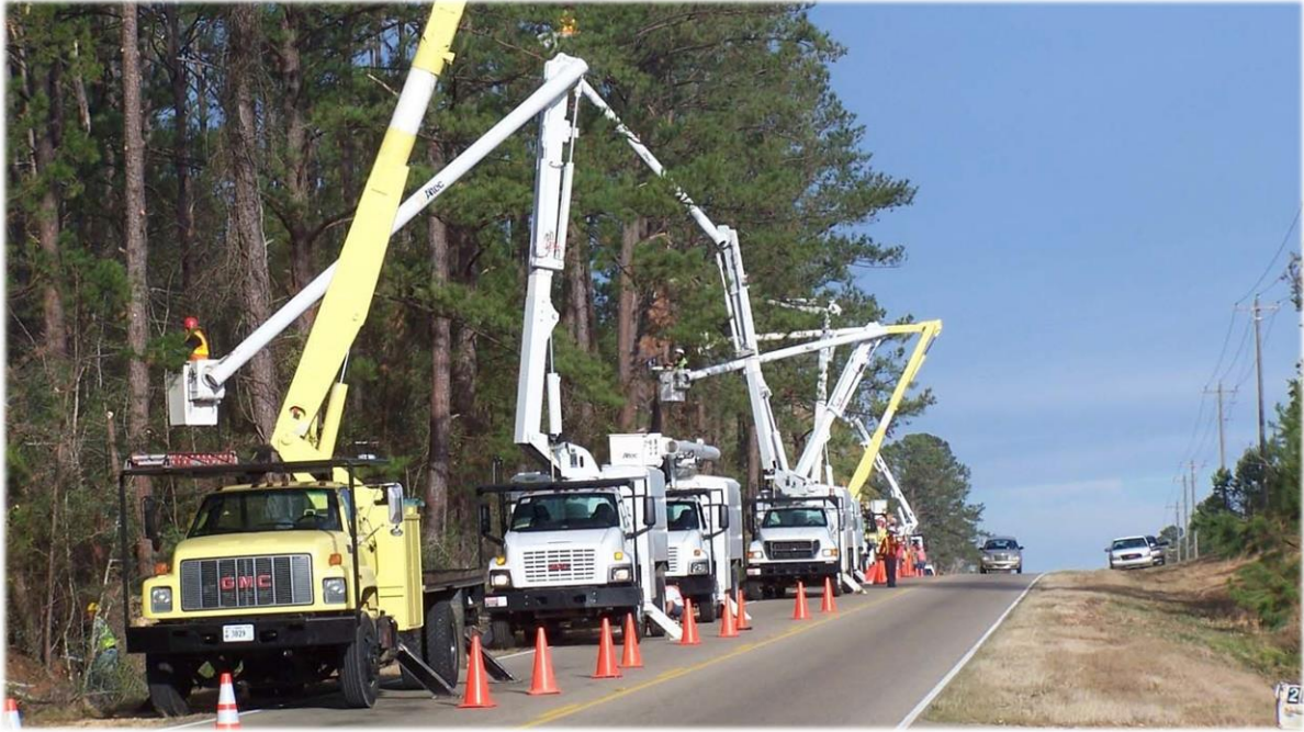
Hazard Tree Removal (Leaner)
