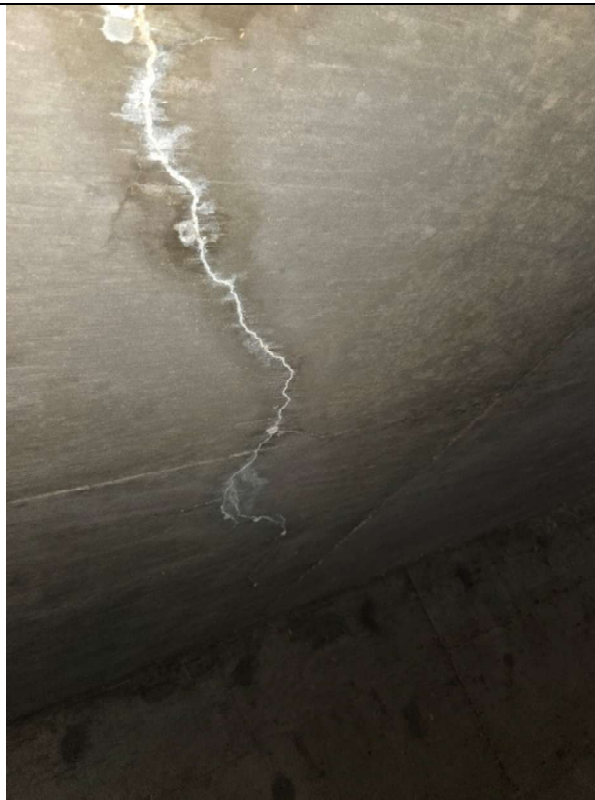
Photograph: 43 Photo of crack in concrete channel.
