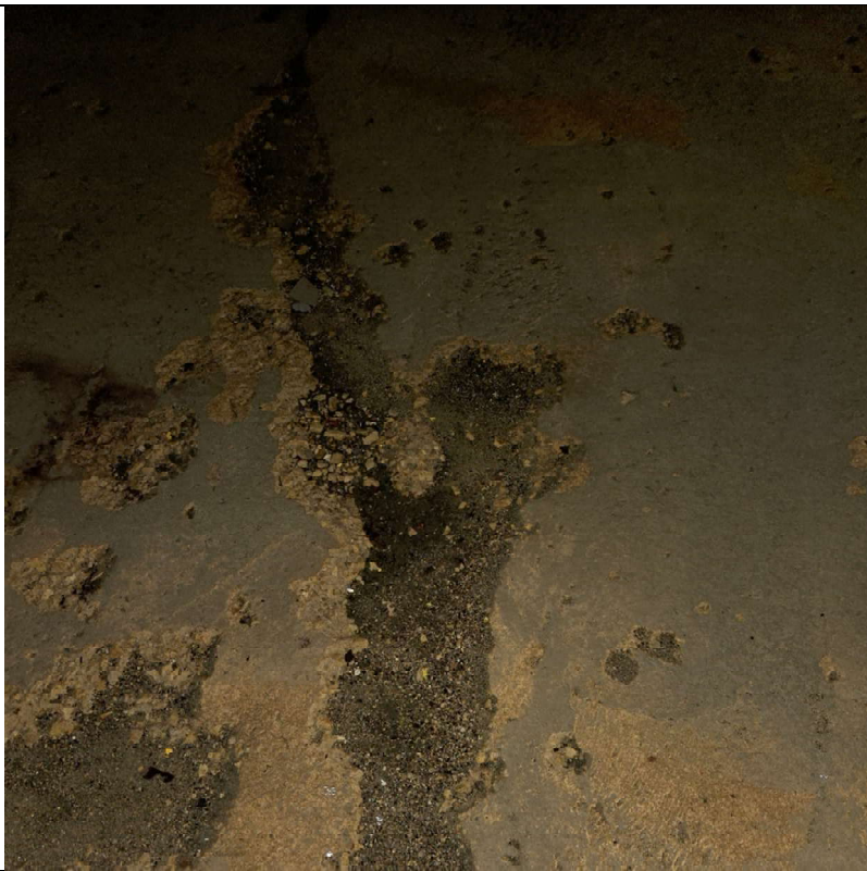
Photograph: 37 | Spalled concrete within channel concrete floor.
