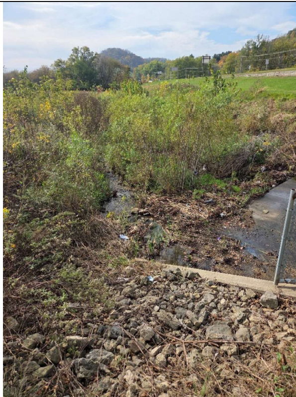
Photograph: 44 Photo taken south the intersection of STH 14 and STH 80. Sediment and vegetation to be removed.
