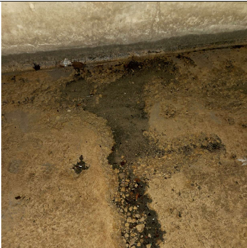
Photograph: 38 | Spalled concrete within channel concrete floor.
