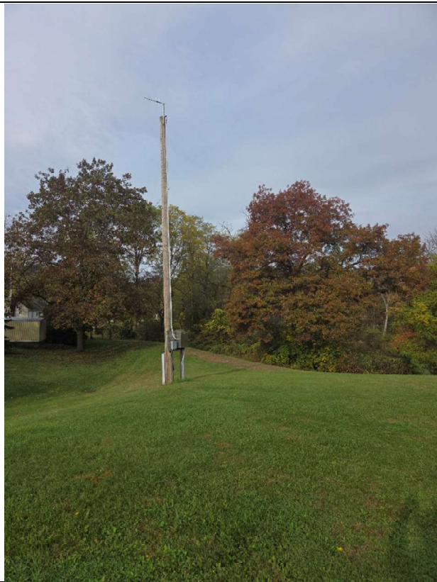
Photograph: 7 | Control panel in good condition.
