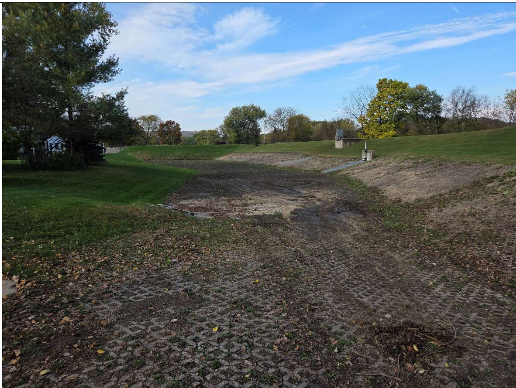
Photograph: 25 Retention basin located south of dike between STH 80 and Church Street. Debris to be removed.
