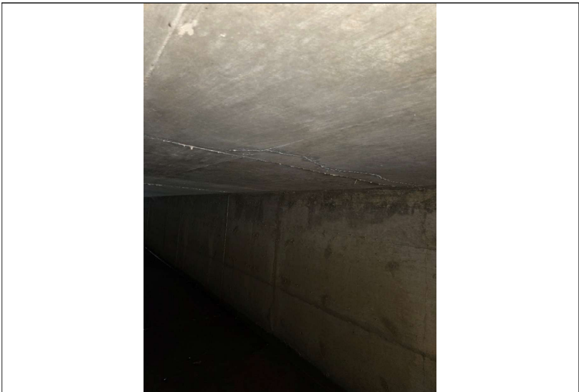
Photograph: 42 | Photo of crack in concrete channel.
