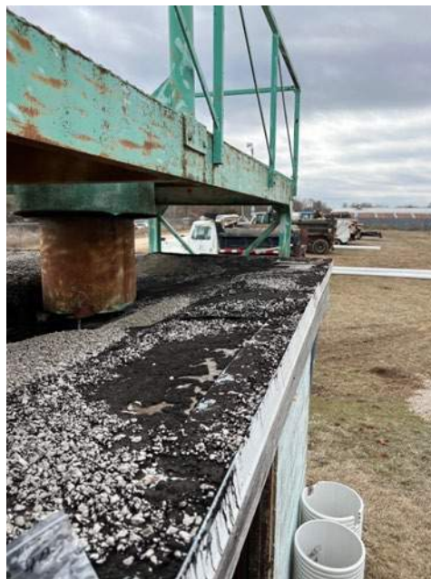
Photograph D-4: Roof of Mini-Storage building has tar on wood – no ACM. Lime paint on metal contains lead.
