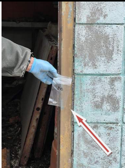
Photograph D-3: Mini-Storage Bldg. Exterior west door to pump room: Sample 3C of Tan/gray door caulking (metal frame to CMU/concrete ext. wall) contains damaged 3-4% chrysotile ACM, Category II, non-friable, damaged. Lime prime paint on frame and CMU walls contains lead.
