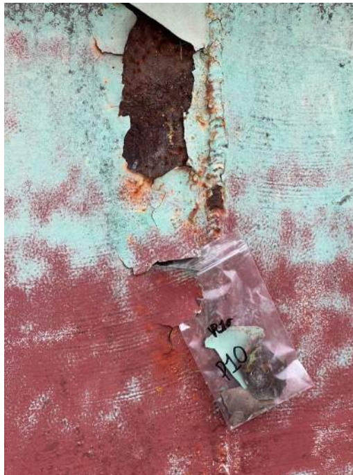
Photograph D-8: Exterior wall of former basin, Sample P10 showing lime paint with red prime contains lead. (Note that all sampled paint contains lead and most also contain cadmium and/or chromium).
