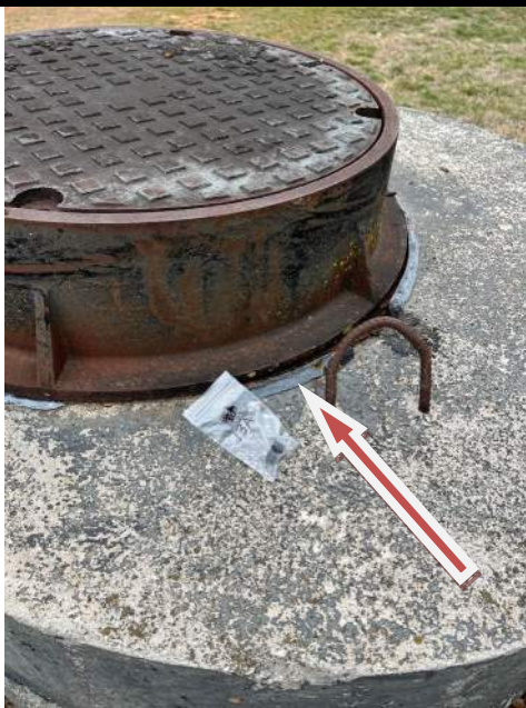
Photograph D-7: Gray/black caulk/sealant (iron to concrete) around top perimeter of manhole riser, west of basin, contains 12% chrysotile ACM, Category I, non-friable in damaged condition. Note that black tar on side of concrete riser and black tar/wrap on nearby pipes do not contain any asbestos.
