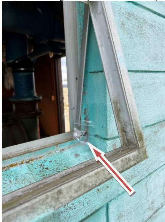
Photograph D-2: Mini-Storage Bldg. Exterior window of pump room, north side: Sample 3B (similar to 3A & 3C) of Tan/gray window caulking (metal frame to CMU/concrete ext. wall) contains damaged 3-4% chrysotile ACM, Category II, non-friable, damaged. Lime paint on CMU walls contains lead.
