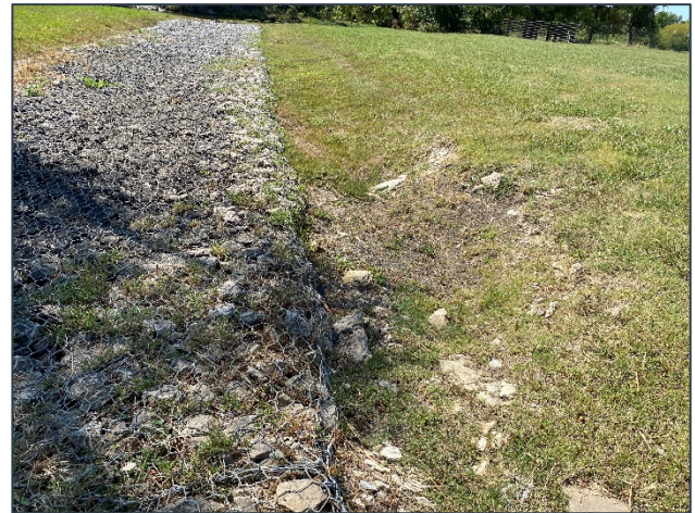
Picture 24. Minor erosion along service spillway
