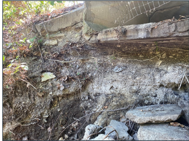
Picture 14. Saturation line 3' below culvert
