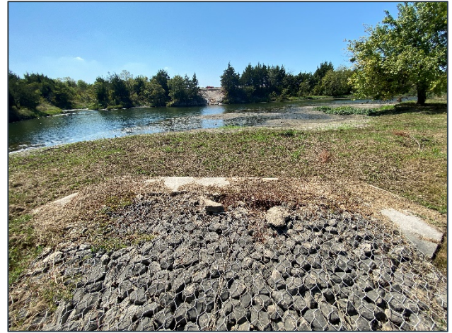
Picture 22. PVC gabion mattress damage upstream end of service spillway
