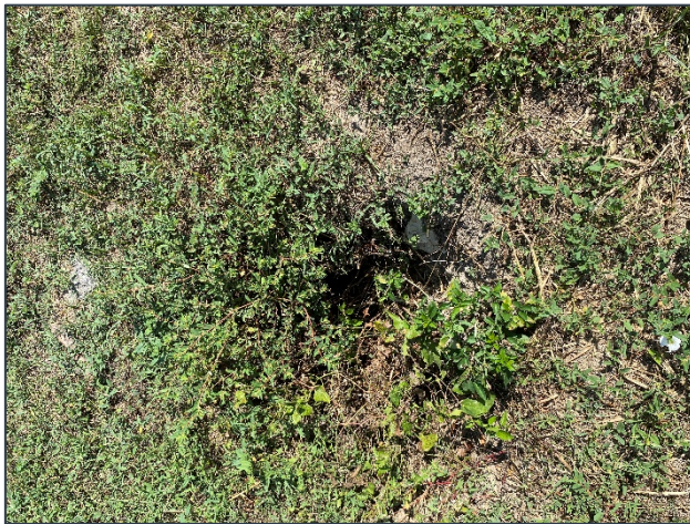
Picture 3: Depression on northwest side of crest
