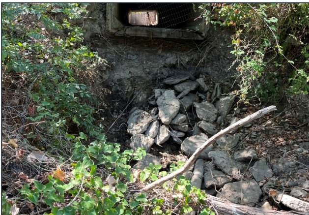
Picture 11. Erosion at toe of culvert downstream embankment
