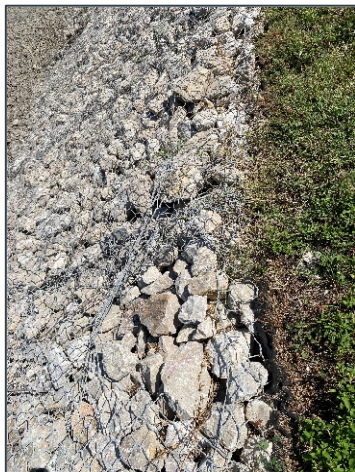
Picture 23. Damaged gabion wire on service spillway
