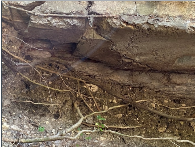
Picture 19. Box culvert reinforcement exposed at downstream end
