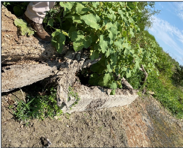
Picture 15. Concrete inlet structure no top grate
