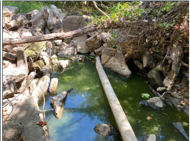
Picture 20. PVC pipe exposed in concrete riprap
