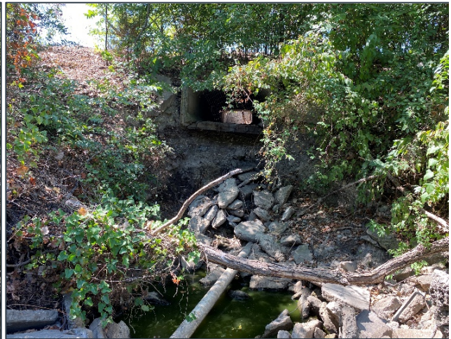
Picture 18. Scour hole at toe of box culvert
