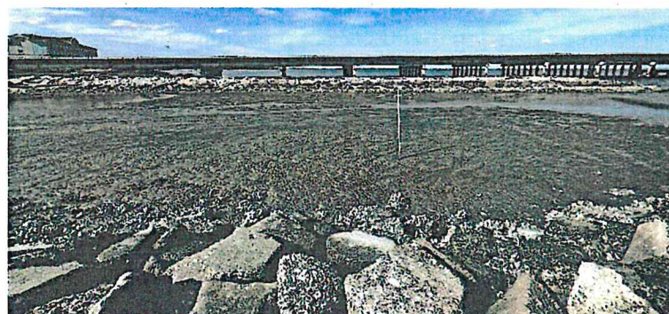
Current silted in condition of entrance channel (very low tide)
