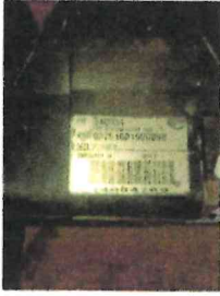
Photo 9 – Description: Pump/value Pic
