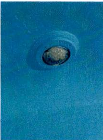
Photo 7 – Description: Light Pic 2
