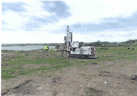
No. 3 View of SB-2 location at the south side of the site.
