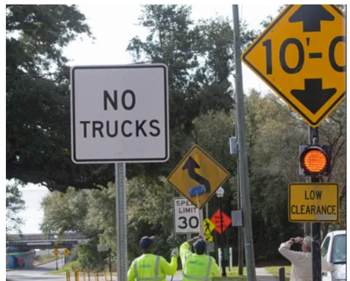
Installation of truck route signage alerting trucks of low clearance. Source: Pensacola News Journal
