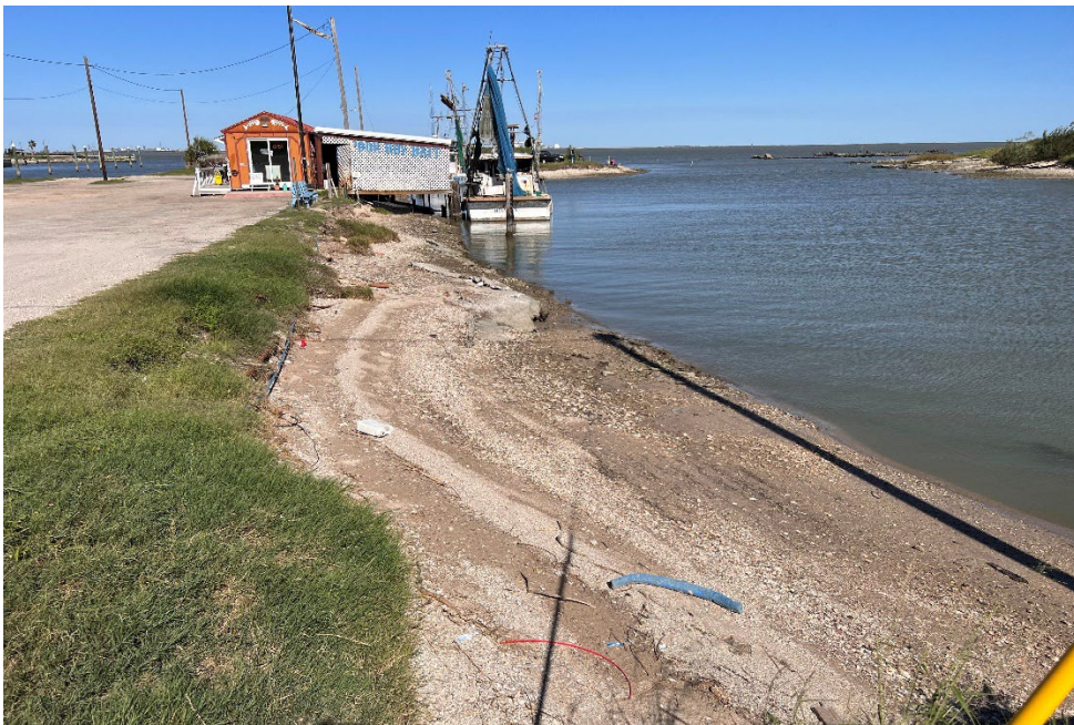
Looking Northeast from Seawall at location of proposed future fishing/crabbing dock and transient boat slips. Photo taken 10.15.2023
