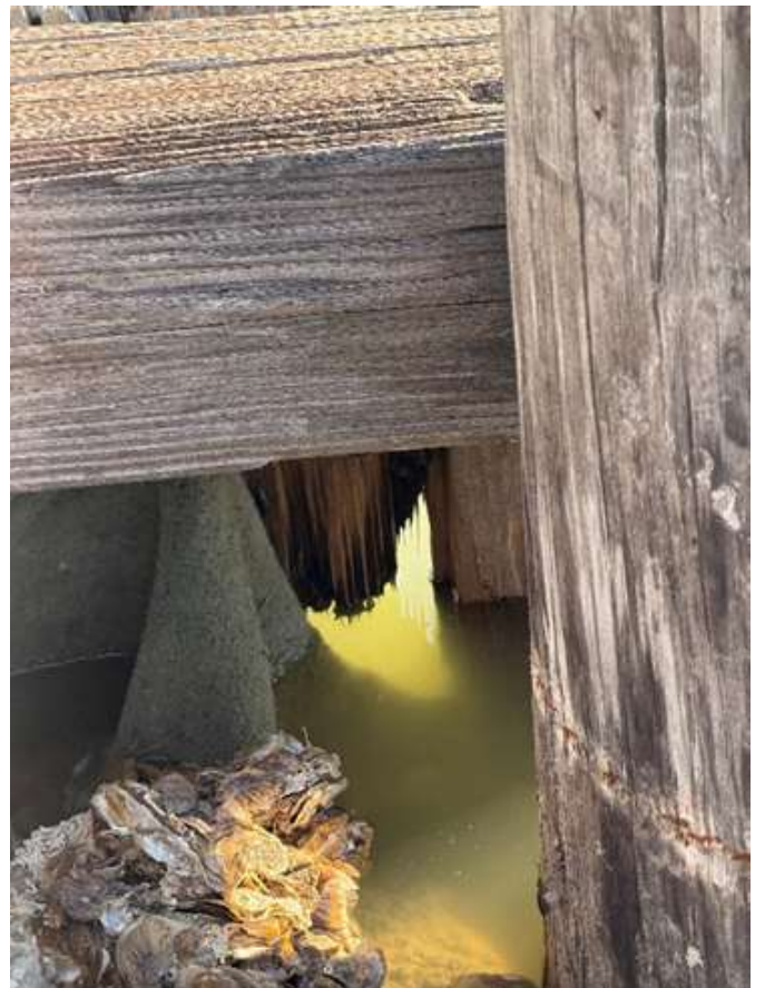
View of deteriorated timber bulkhead at the terminus of the bulkhead.
