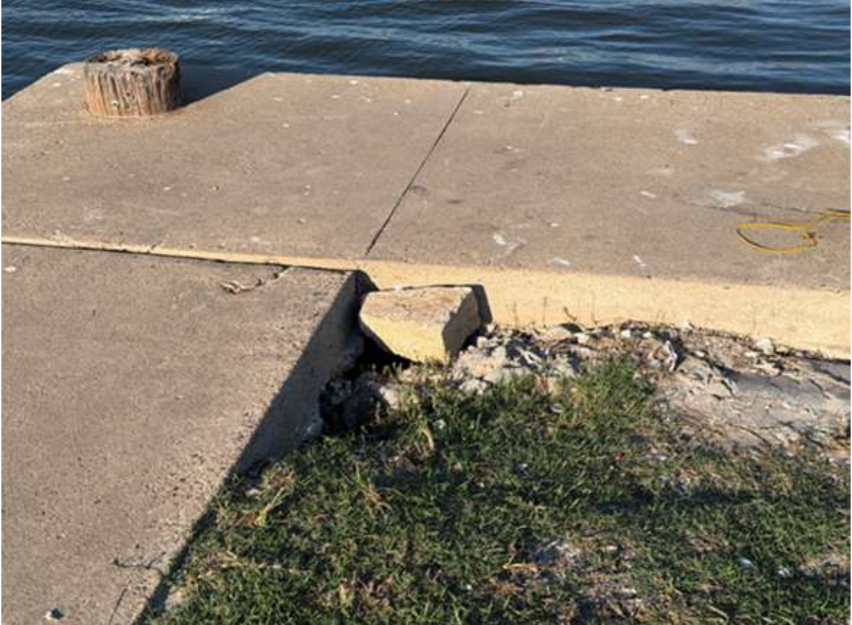
Evidence of subsidence (washout) underneath the concrete cap/walkway at the northeast corner of the boat ramp. (Oct. 12, 2026)
