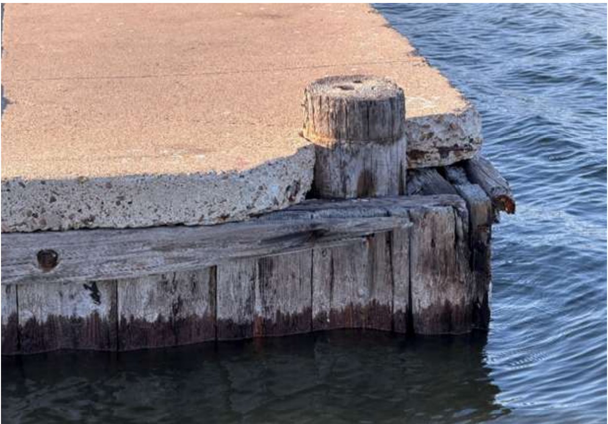
Deterioration of the northwest corner of the boat ramp.
