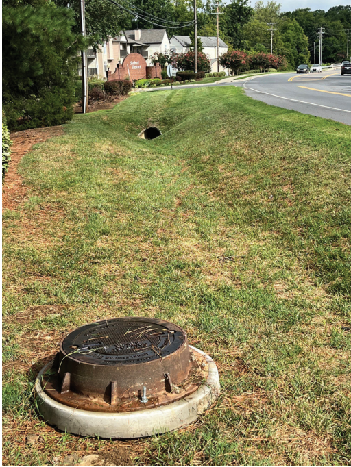
Sewer line manhole and side drain culvert at the alignment of the new sidewalk looking north towards Sable Point Drive.
