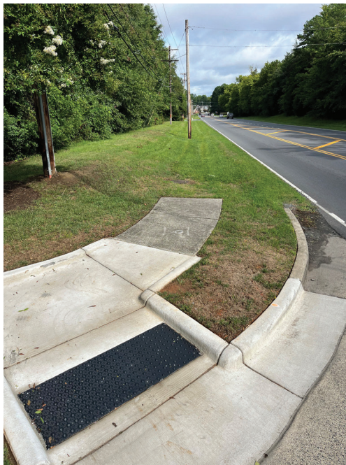
South end of the project looking north where the new sidewalk will be connected to the existing sidewalk at the car wash property.
