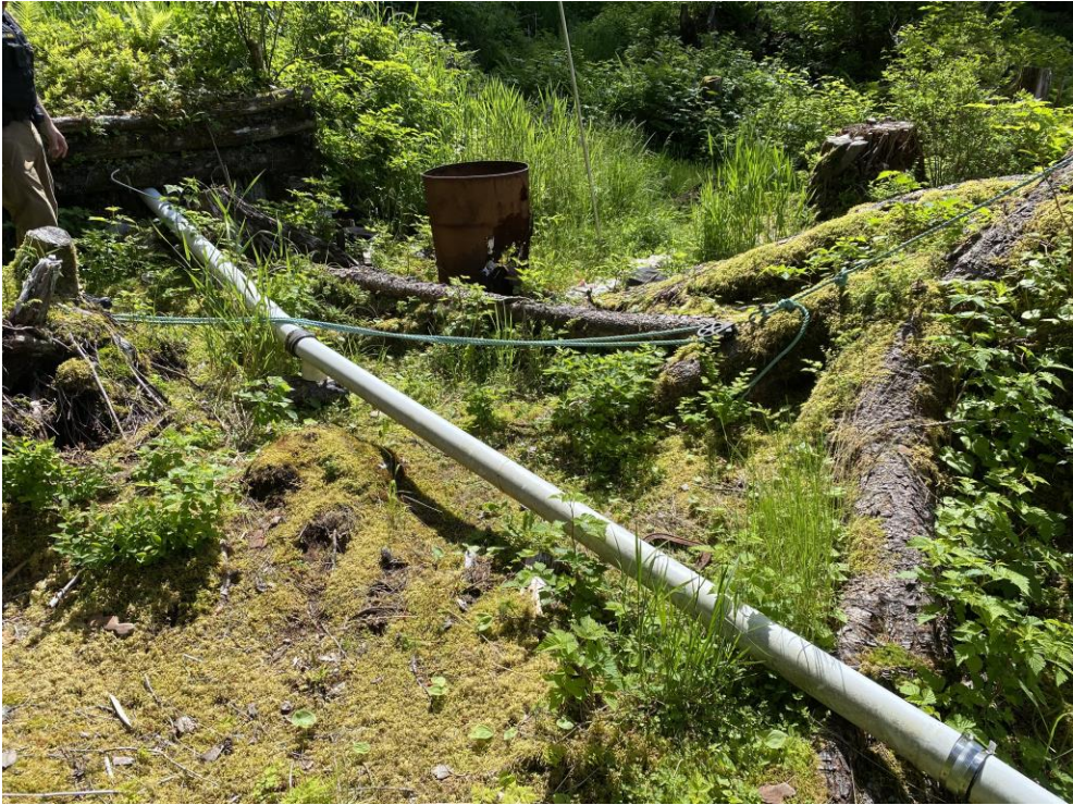
Pipe connected to septic tank.
