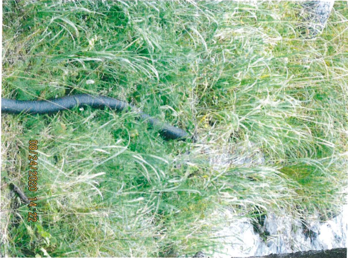
Photo showing discharge of corrugated pipe to a surface water drainage adjacent to beach of Wrangell Narrows.
