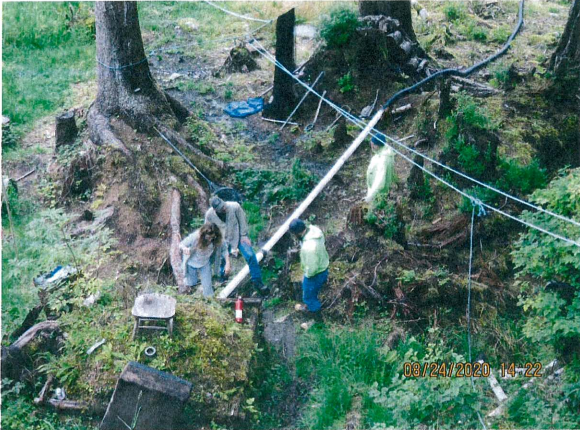
Photo showing piping route and connections to septic tank.
