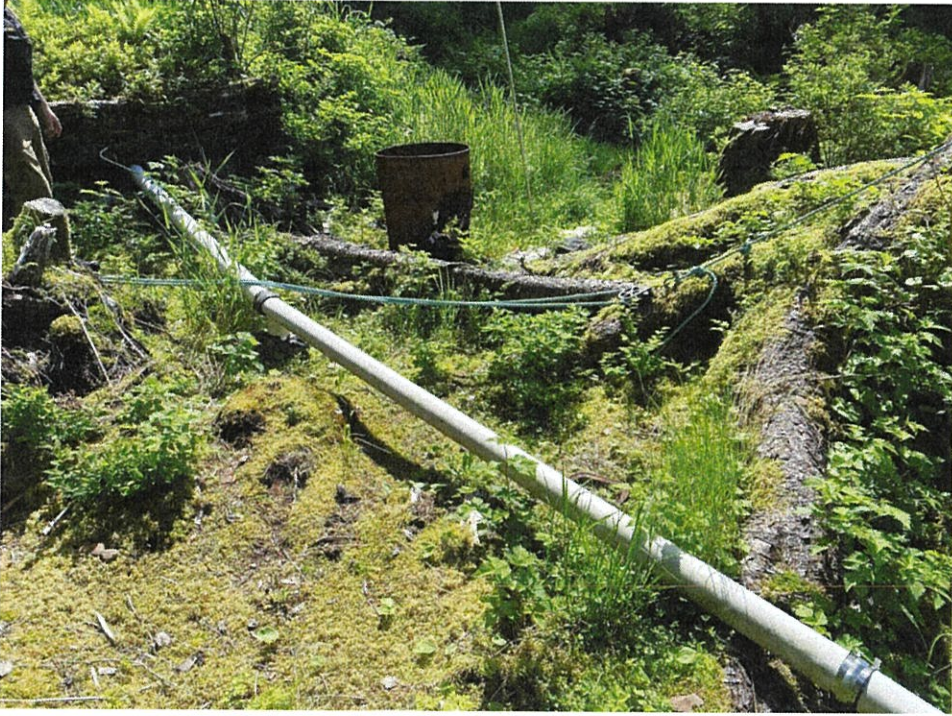
Pipe connected to septic tank.
