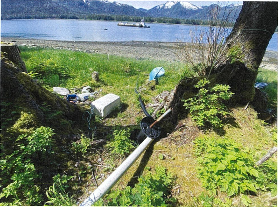
Pipe from septic tank going to beach.
