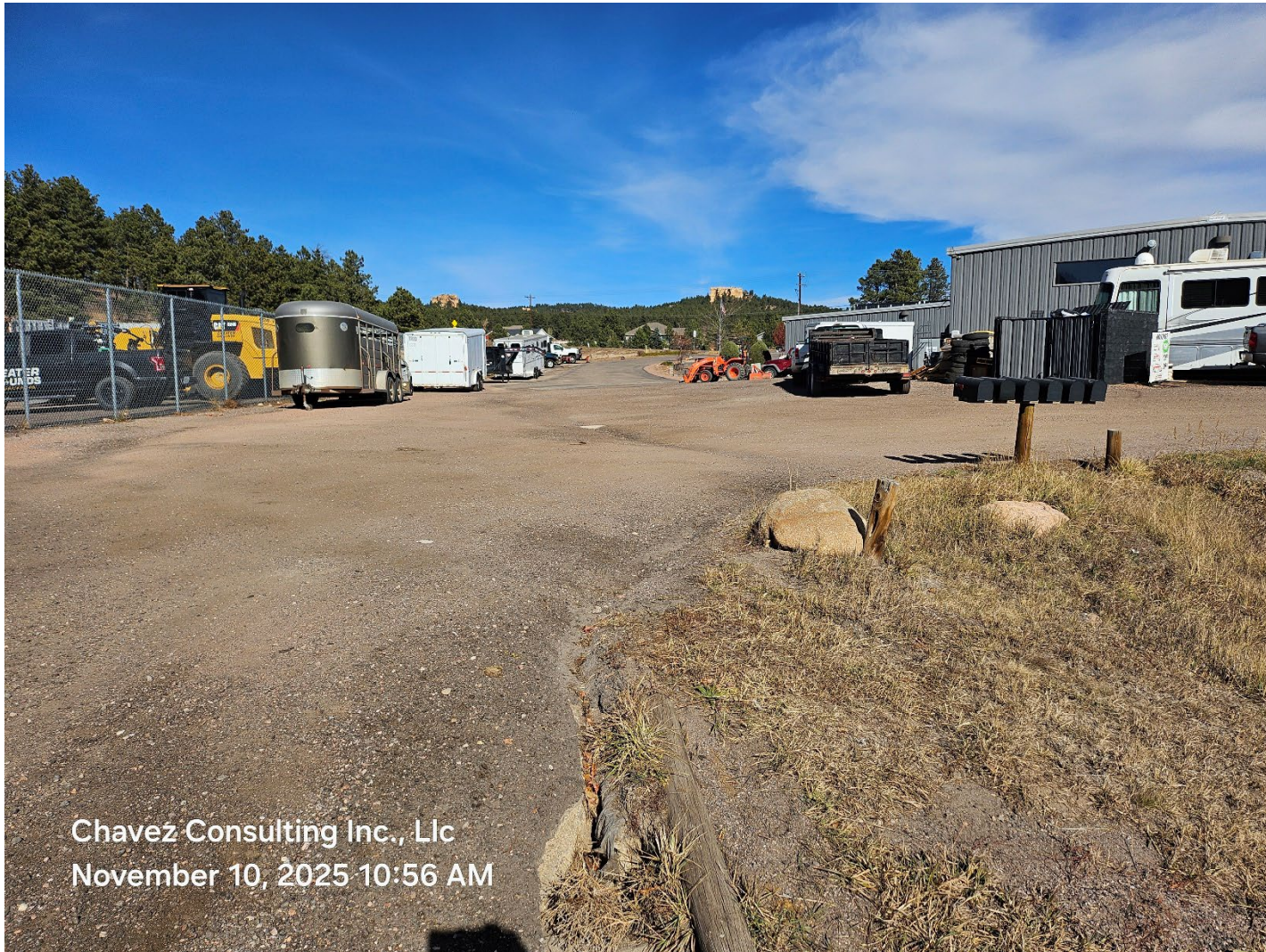
Figure 7. Site Drainage: runoff is bypassing existing extended detention basin.
