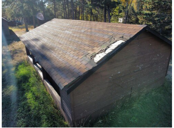
Replace damaged OSB.
