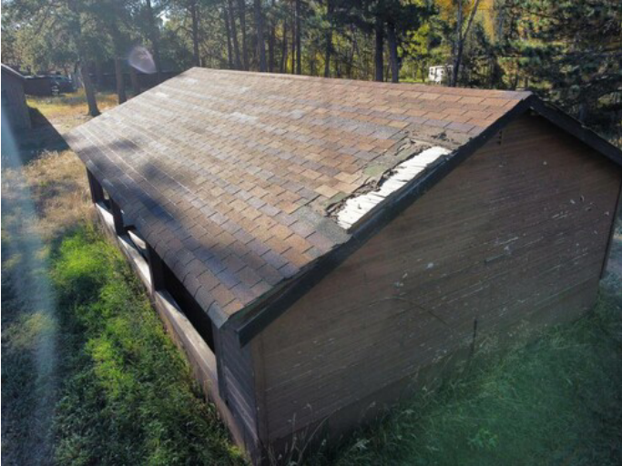
Replace damaged OSB.
