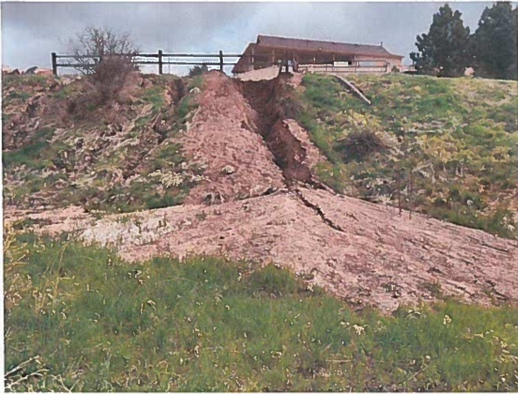
Figure 4: Erosion below the intersection of Lake Ave and Cathedral Ave after a rainstorm, taken from the Santa Fe Trail May 15, 2024
