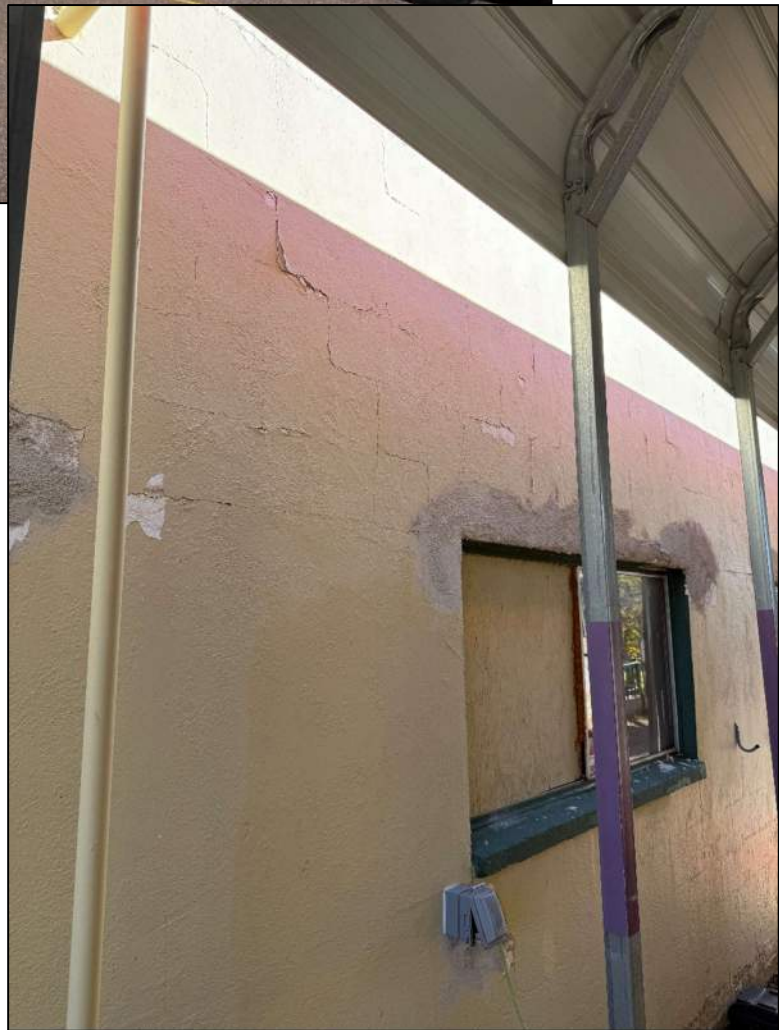
Photo 2: South wall looking northeast under the fire truck roof structure. Notice cracking in plaster defining the 8"x16" CMU blocks. Lots of plaster patches were presents.
