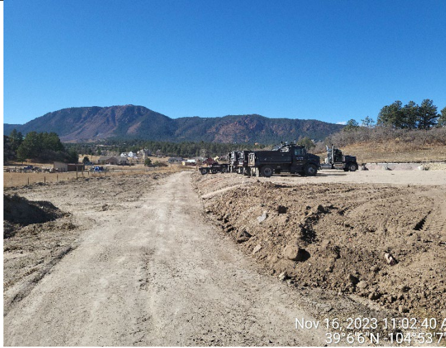
Figure 1. Northeast property corner, looking south down east property line. No stormwater control measures in use.
