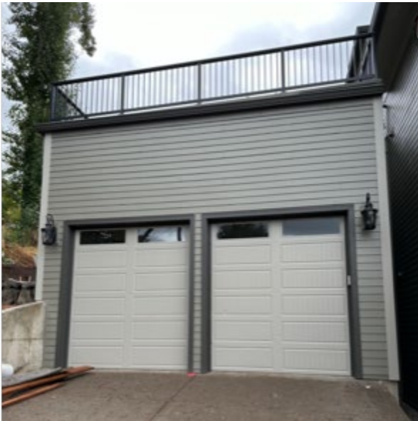
Photo of garage showing existing garage railing with use of Alumarail by Precision Rail
