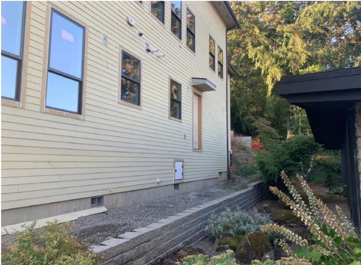
Figure 4 Existing condition of side elevation showing unpermitted CMU wall. - September 20, 2022 . CMU wall has been removed as of November 15, 2022
