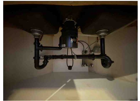
Kitchen Sink Drain/Disposal
