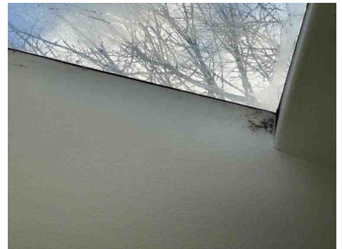
Black Mold Bathroom Skylight
