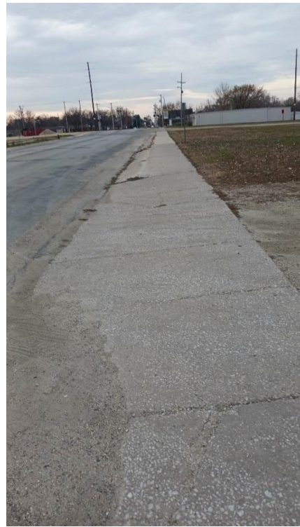
Cross slope greater than 2%
