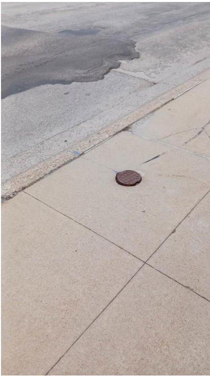
Protruding water valve
