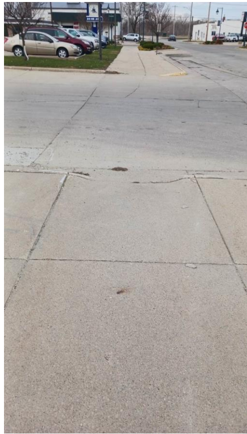
Non-compliant pedestrian ramp
