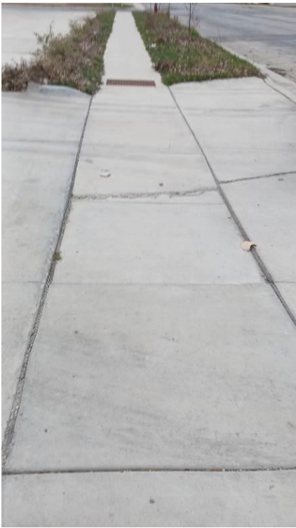
Crack with vertical displacement
