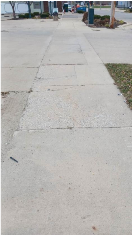
PCC displacement greater than 0.25"
