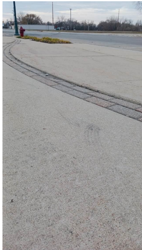
Pavement settling along paver band
