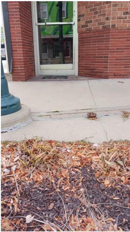
Protruding curb stop
