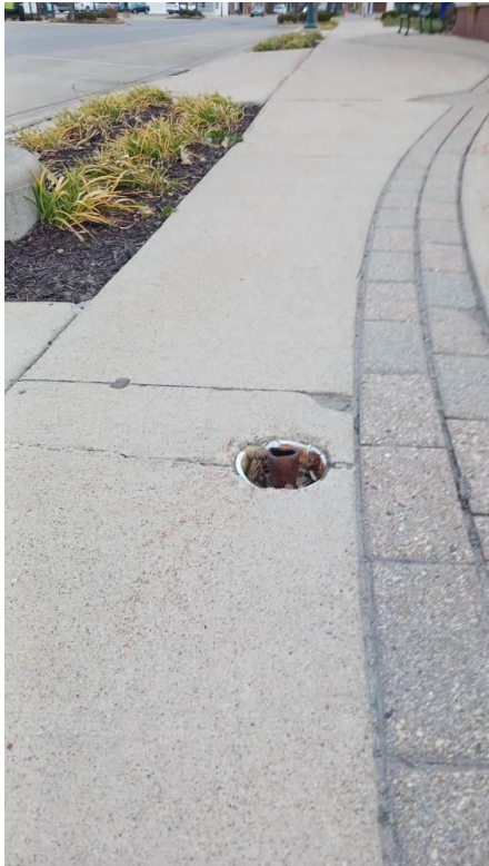
Curb stop box protruding with opening around box
