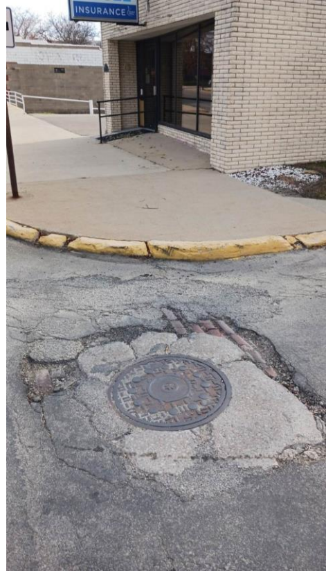
Non-compliant curb ramp
