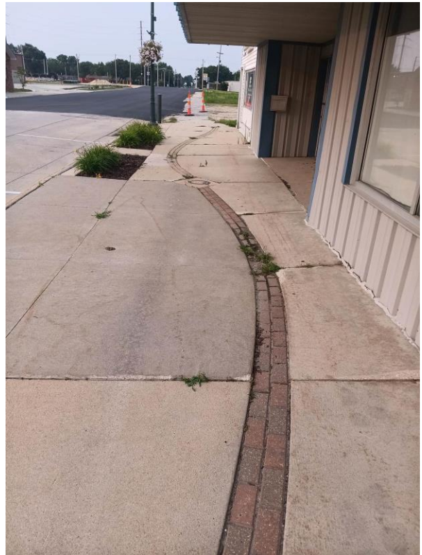
Vegetation in joints
