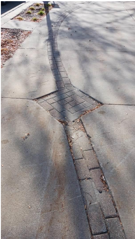
Settled pavers and diamond
