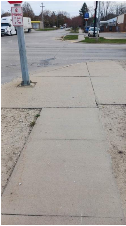
Non-compliant curb ramp
