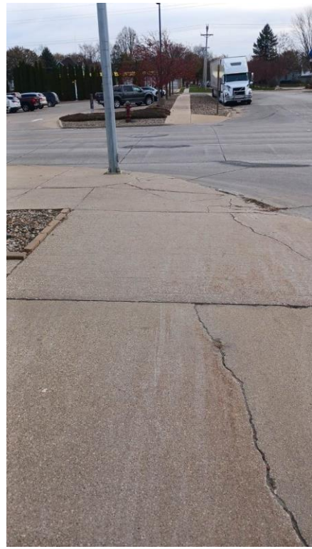
Non-compliant curb ramp
