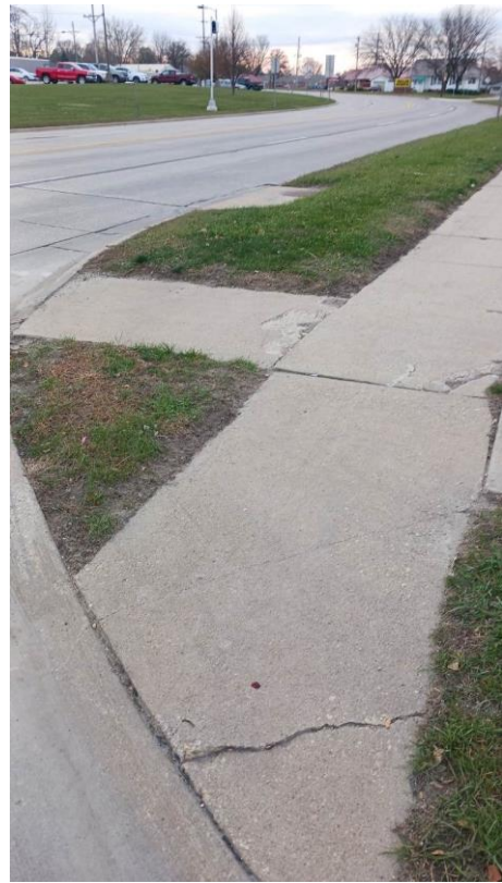
Non-compliant pedestrian ramp
