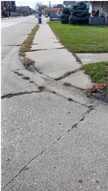
Non-compliant pedestrian curb ramp
