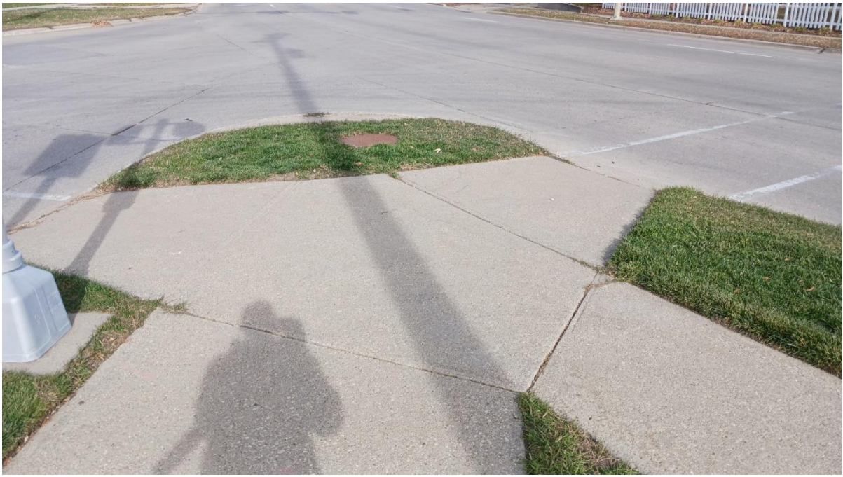
Non-compliant pedestrian curb ramp
