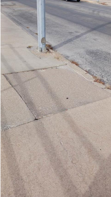
Settled PCC panel
