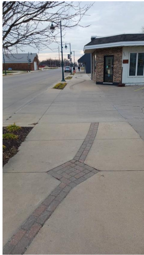
Paver settling greater than 0.25"
