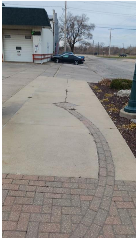
Cross slope greater than 0.25"
