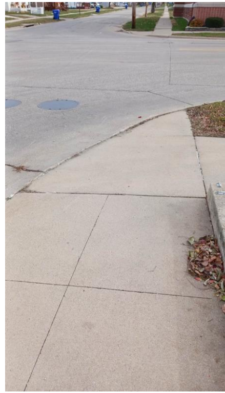
Non-complaint pedestrian curb ramp
