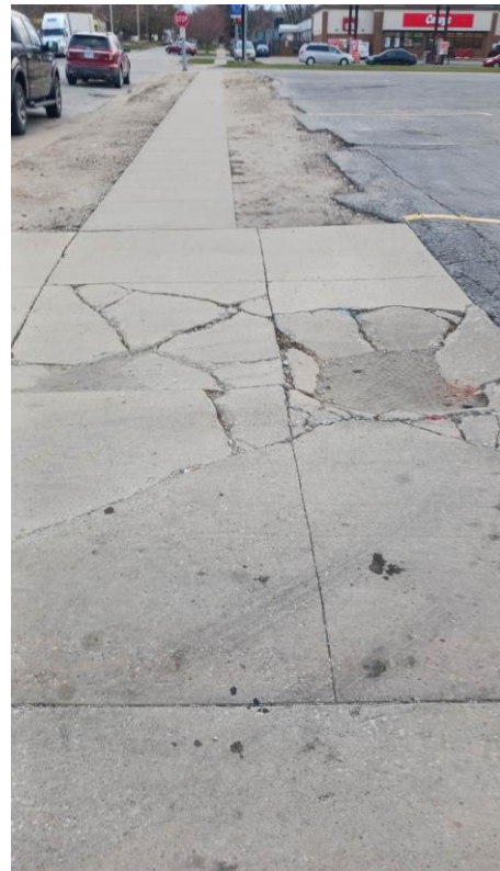
Severely broken PCC
