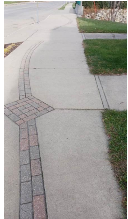
PCC displacement across paver band
