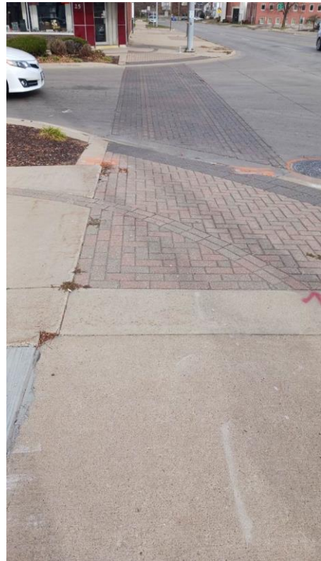
Settled pavers around curb ramp perimeter
