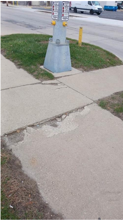
Broken/missing PCC with vertical displacement greater than 0.25"
