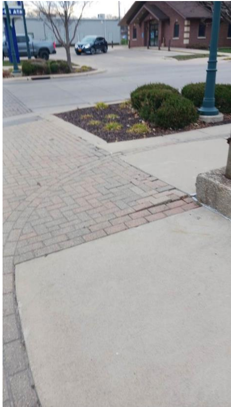
Heaving pavers with vertical displacement greater than 0.25"
