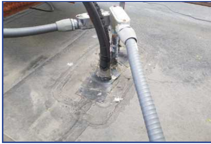
Section B - Deficiency #1 Lines through roof are electrical taped
