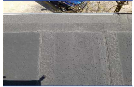
Section A - Deficiency #3 Open or Missing T-Joint patches
