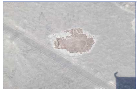
Section A - Deficiency #5 Failing caulking
