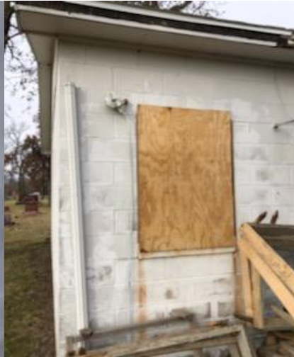
WINDOW BOARDED UP
