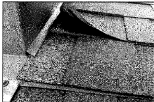
Section B - Deficiency #5 Poorly installed flashing
