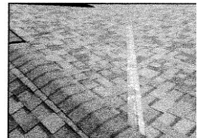
Section B - Deficiency #3 Deteriorated valley tin
