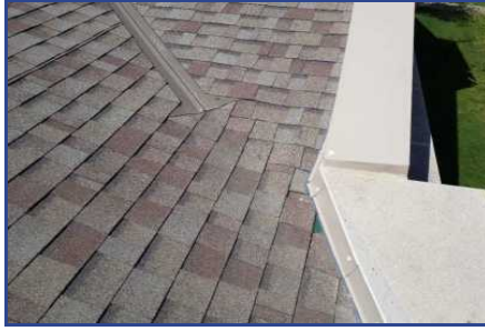
Section B - Deficiency #7 Roof decking corroded, deteriorated or deflected
