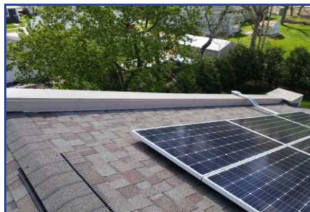
Section B - Deficiency #1 Improper installation of shingle step flashings
