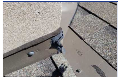
Section A - Deficiency #1 Improperly installed step flashing along Gable wall
