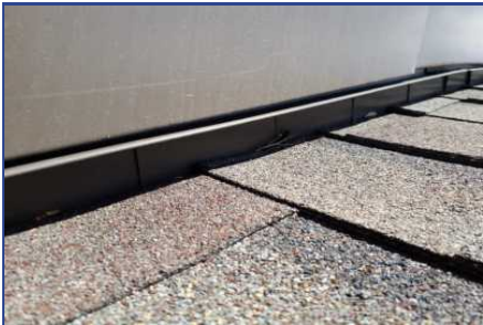
Section A - Deficiency #1 Improperly installed step flashing along Gable wall
