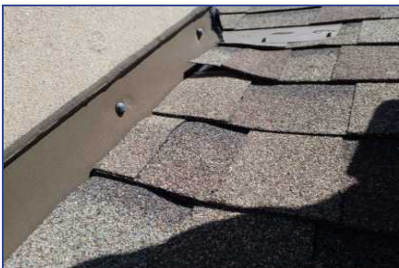
Section A - Deficiency #1 Improperly installed step flashing along Gable wall Improperly installed step flashing along Gable wall
