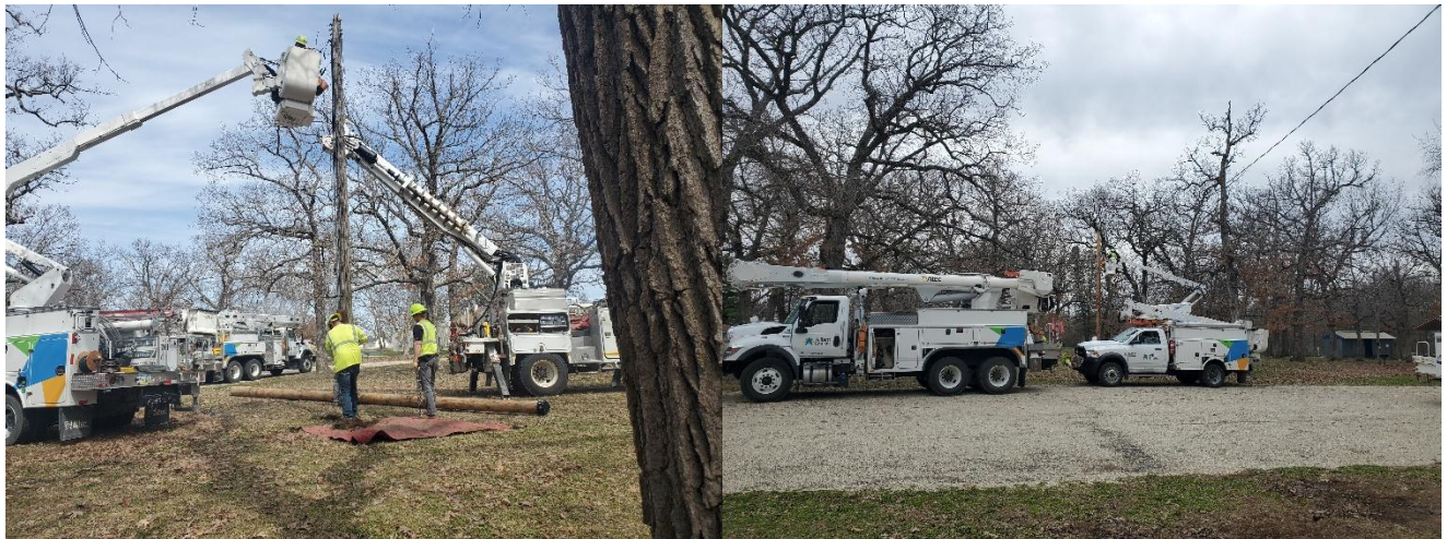
UTILITY POLES – CITY PARK
