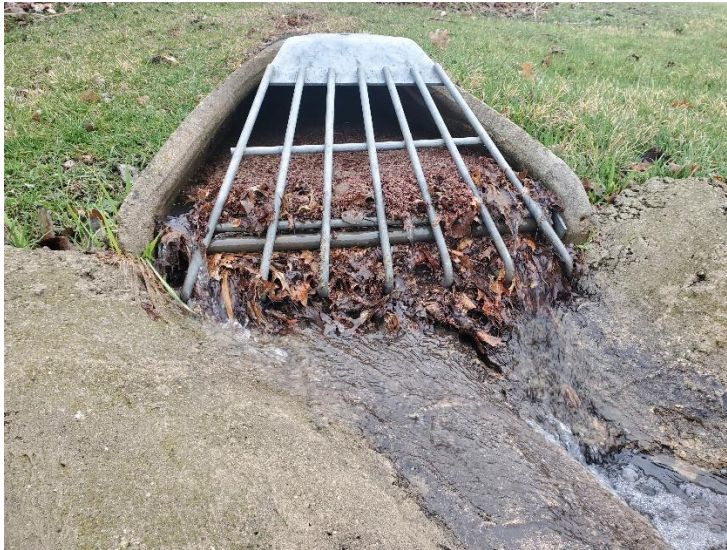
PLATT PARK INTAKE
