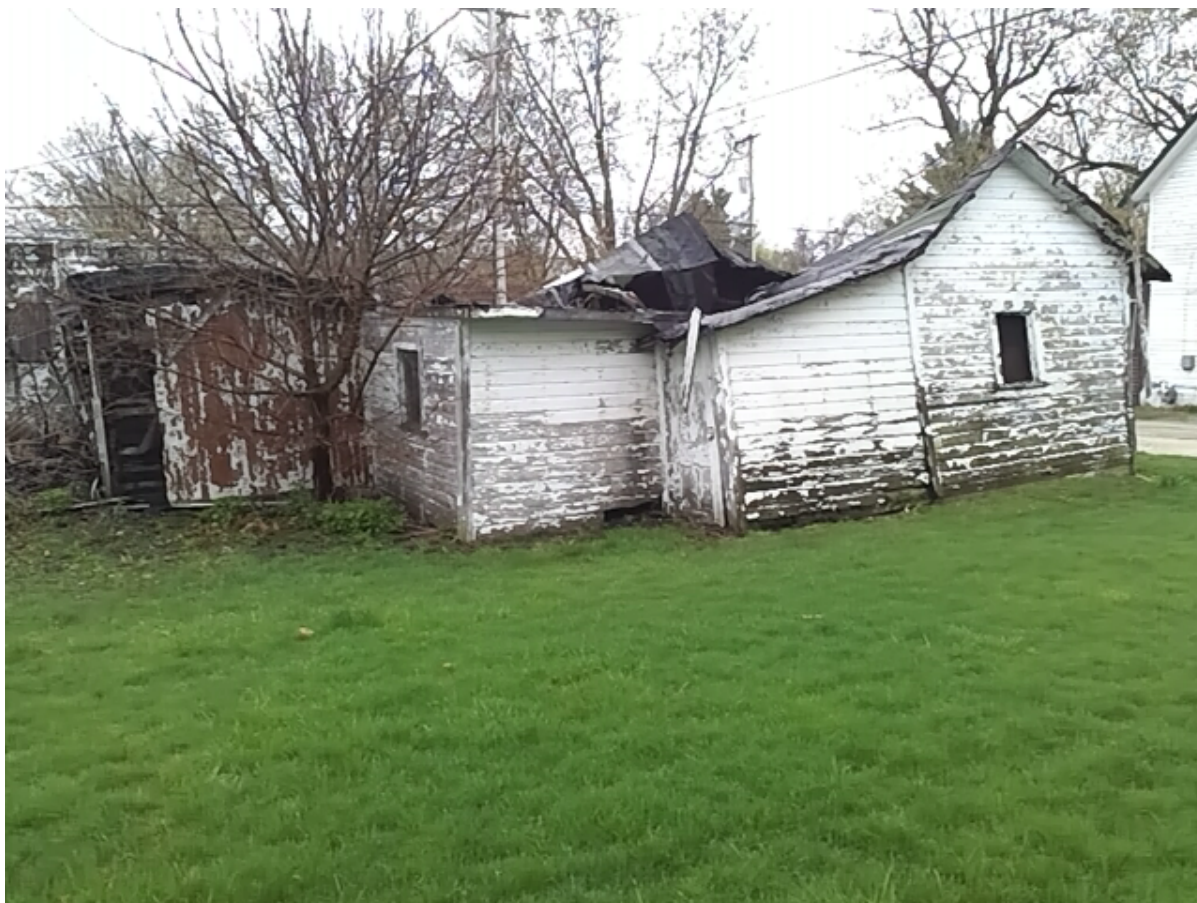
Photo: Collapsed Structure
