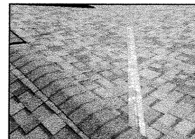
Section B - Deficiency #3 Deteriorated valley tin
