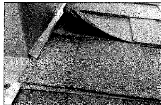
Section B - Deficiency #5 Poorly installed flashing
