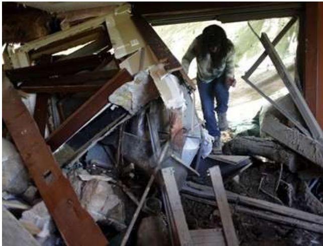
Figure 28. Landslide Damage to a Historic Jordan Brewery (Feyder, 2014)
