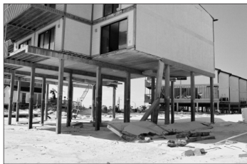
Figure 16. Shore-perpendicular reinforced masonry wall failed and collapsed into the foundation of an adjacent building, contributing to failure of the corner foundation piling and pile cap/beam.
