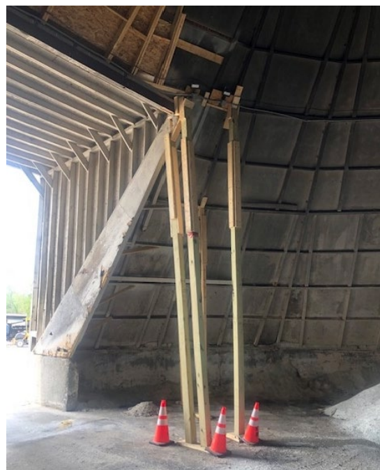
Damaged Framework and Entrance
