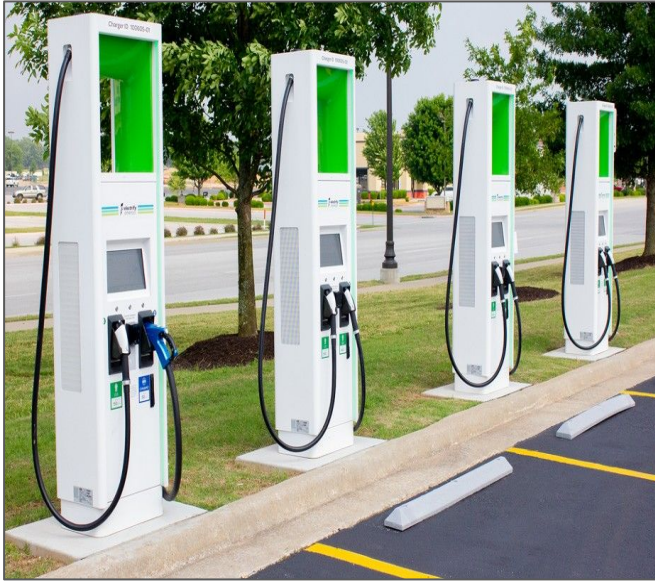
EV Charging Stations
