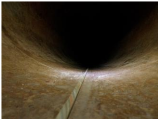
AFO cable in pipe
