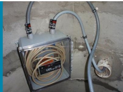
AFO Cable splice point
