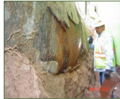
Inspecting the damage
