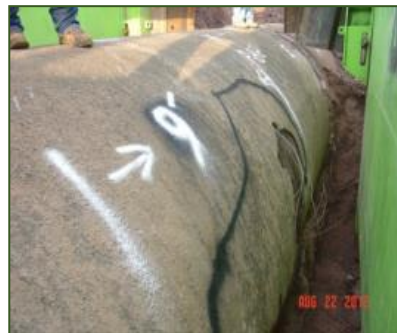
Damage concentrated in 9' section
