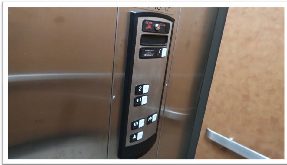
Photograph 16: Typical view of elevator controls
