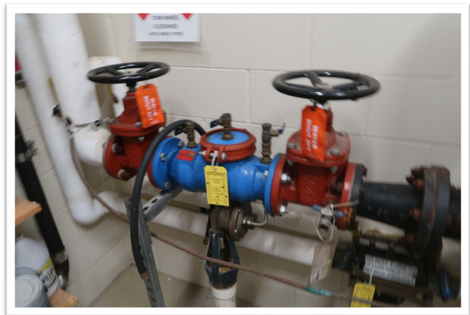
Photograph 22: Typical view of backflow preventer
