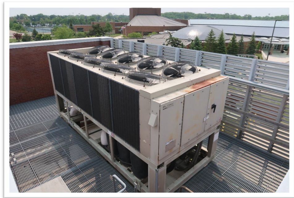
Photograph 18: Typical view of 60 ton chiller
