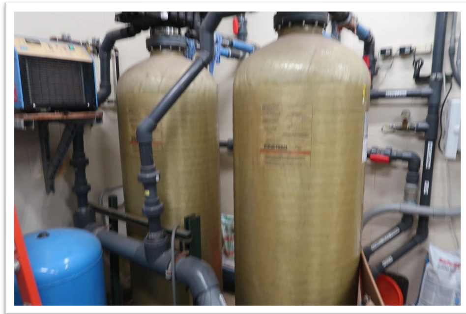
Photograph 20: Typical view of irrigation system sand filters
