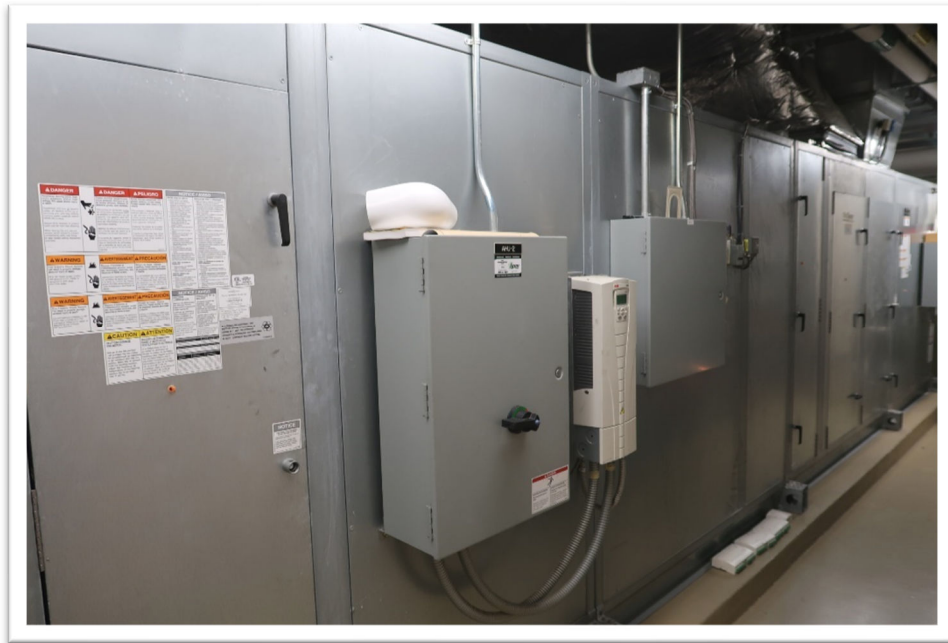
Photograph 19: Typical view of air handler
