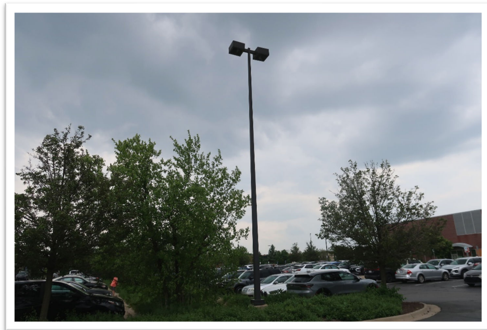
Photograph 34: Typical view of pole light
