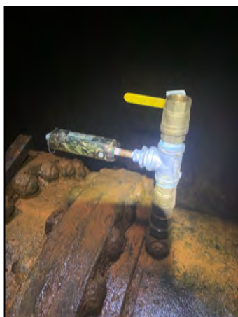
Figure 4.1: TPM mounted downstream of NV-04.
