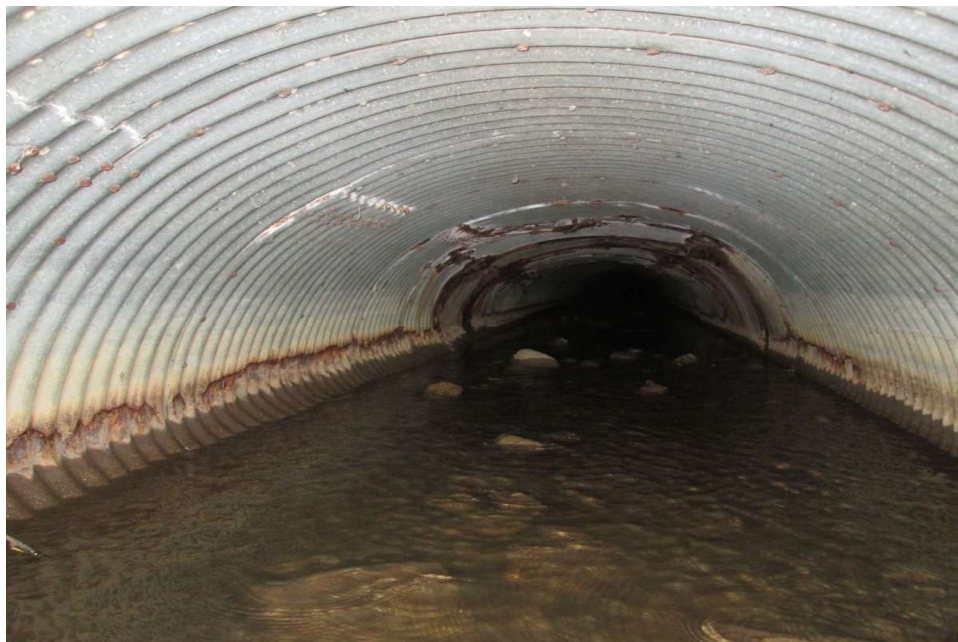
North pipe damage
