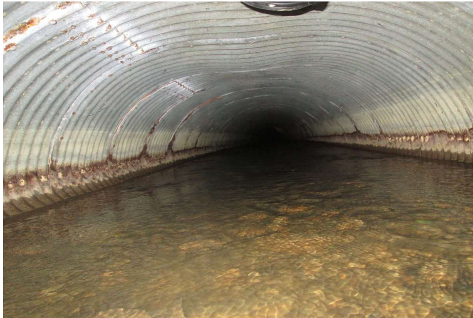
South pipe out of round
