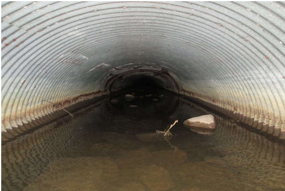
North pipe damage
