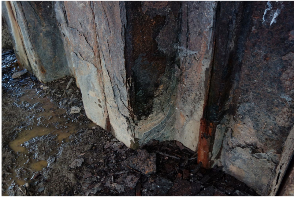
North Abutment Sheeting Section Loss and Rusting
