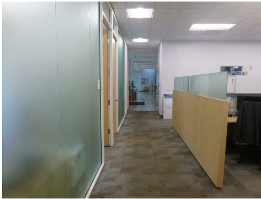
2nd View Office LED Lighting
