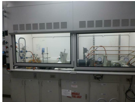
Typical LAB Hood with Sash Control
