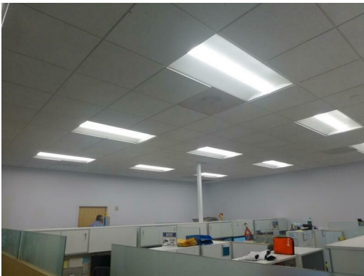
Office LED Lighting-Typical
