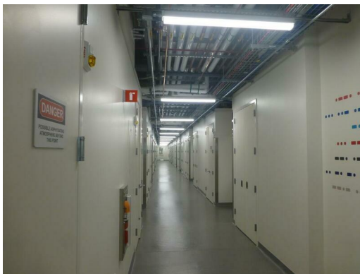
Corridor LED Lighting
