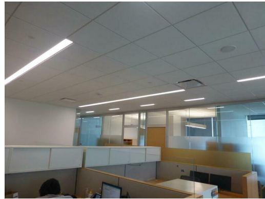
Corporate Office LED Lighting
