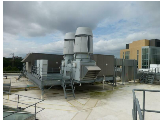
Strobic Fans and Rooftop
