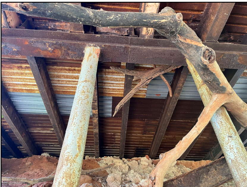
Figure 5 – Rust and Pitting in the Bottom Flange of Pier Cap
