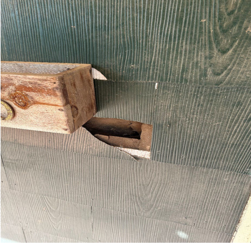
Damaged siding on porch
