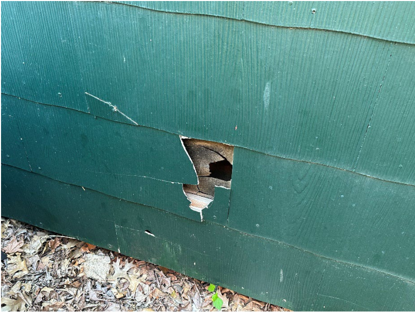
Damaged siding on north side of home
