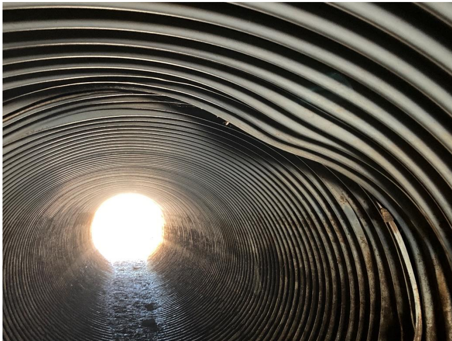
E. pipe 20.5' from north end 3" deflection
