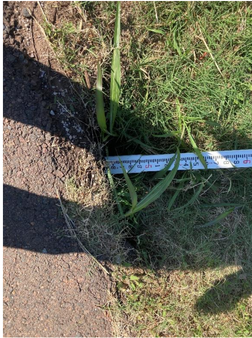
Erosion 4.5' under asphalt with 2' deep void
